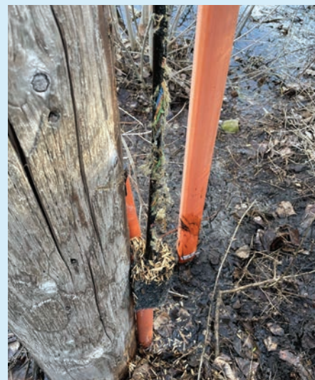
Squirrel-damaged fiber (photo courtesy of Nsight)
