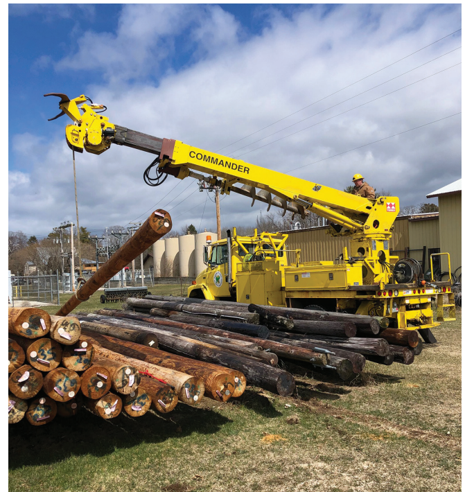
Your cooperative crew continues to work to make sure the lights stay on.
