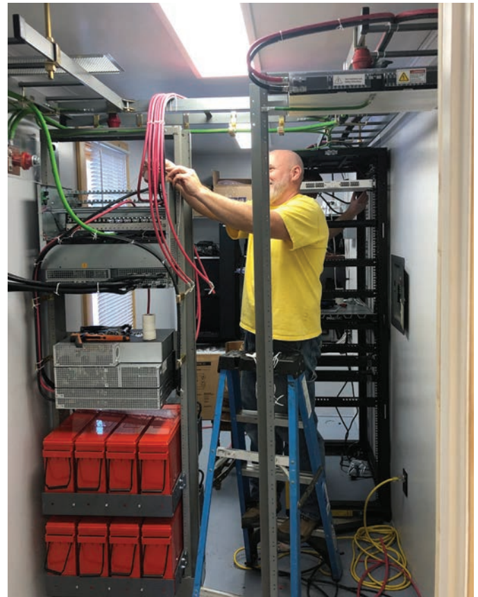
Leon and Andrew Backos (father and son) of RTS install DC (Battery) powerplant and route wiring to server racks.
