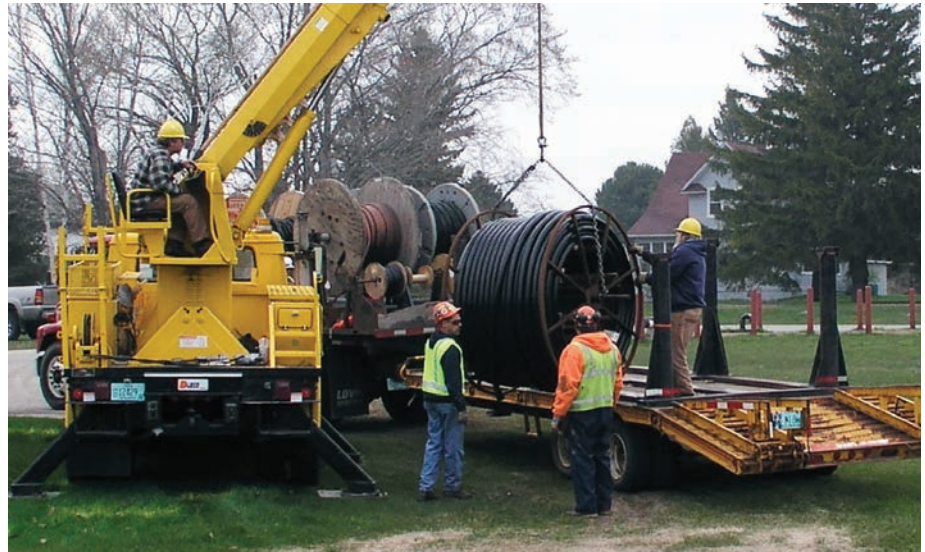
Randy and Don with Arby crew loading cable in conduit for underground replacement in 2004.
