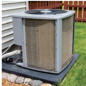
A clean outdoor AC unit (left side) will work much more efficiently than a dirty one (right).
