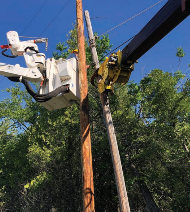
Mike Jorgenson stabilizes the failed pole while Don Johnson transfers a Frontier pole attachment to the new pole. Note that the conductors have already been relocated and this work was done with the power down. The failed pole was installed in the mid 1960s.
